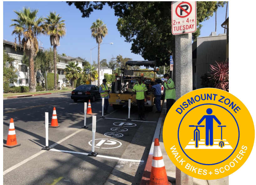
The City of Santa Monica installed parking zones and sidewalk medallions to encourage better parking behavior and reduce sidewalk riding conflicts. Source: City of Santa Monica
